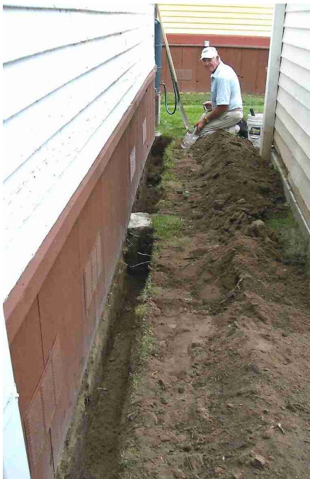
Tom McDonnell shown trenching around the historical society buildings. This is part of the ongoing maintenance that never seems to end. Thanks, Tom.
